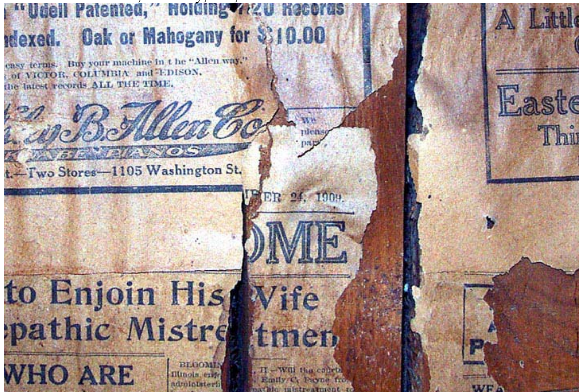
1909 Newspaper, used as insulation, 2 nd floor, 1102 10 th Street
